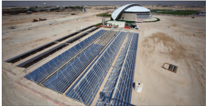
▲ The CSP solar collector array at the showcase stadium.
