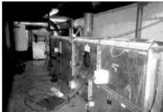
42 m 2 of solar collectors supply a desiccant cooling system in Lisbon/Portugal, which provides air conditioning for 11 office rooms. A monitoring of this system will be carried out in Subtask D.
